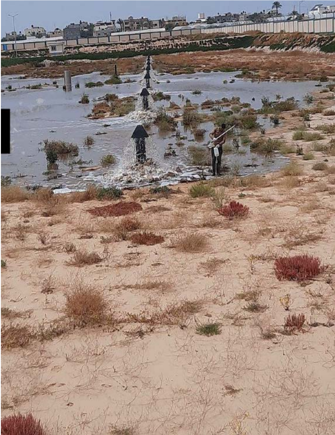
Treated Effluent Pumped to the Infiltration Basins up to June 2020
