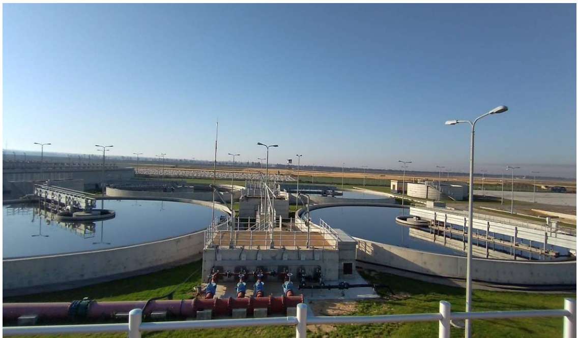
Clarifiers Under Operation up to June 2020
