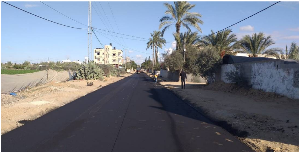
Asphalt Work in Road No.14 in Al Fukhari in December 2019 up to completion in January 2020
