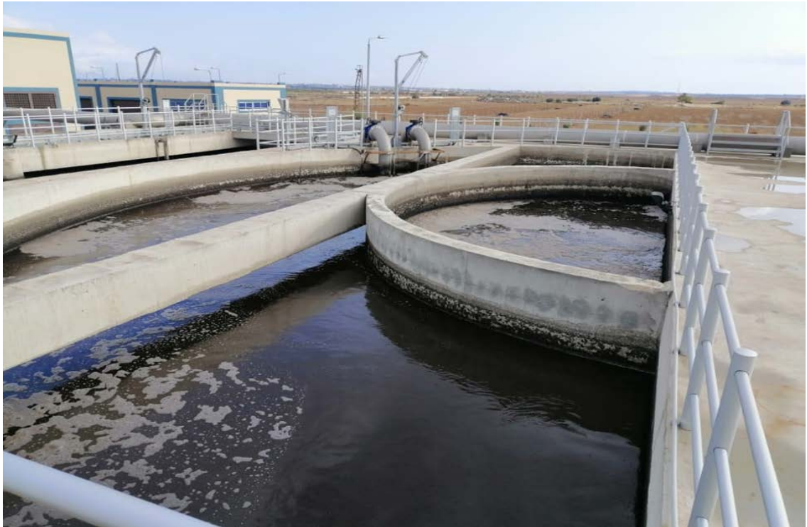
The Aeration Tank Under Operation up to June 2020
