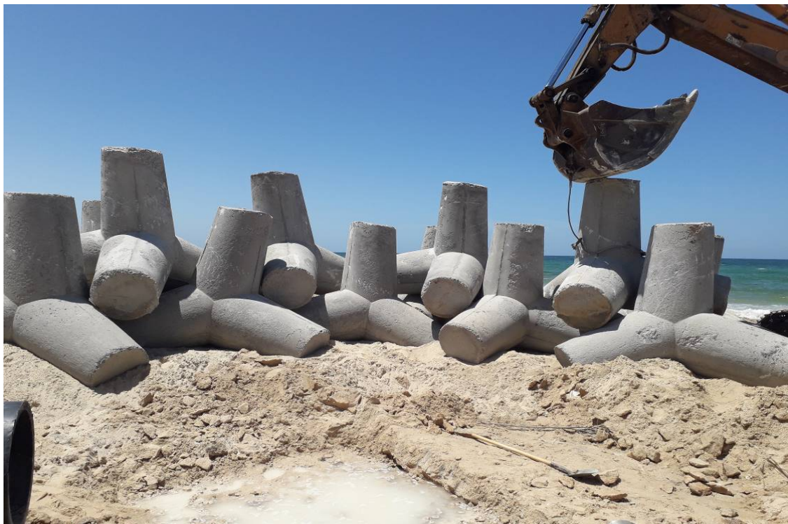
Installation of HDPE Pipes and Interlocking Blocks Tetrapod Shape for Sea Outfall for the Effluent Pressure Lines (CMWU Package) up to Completion in June 2020
