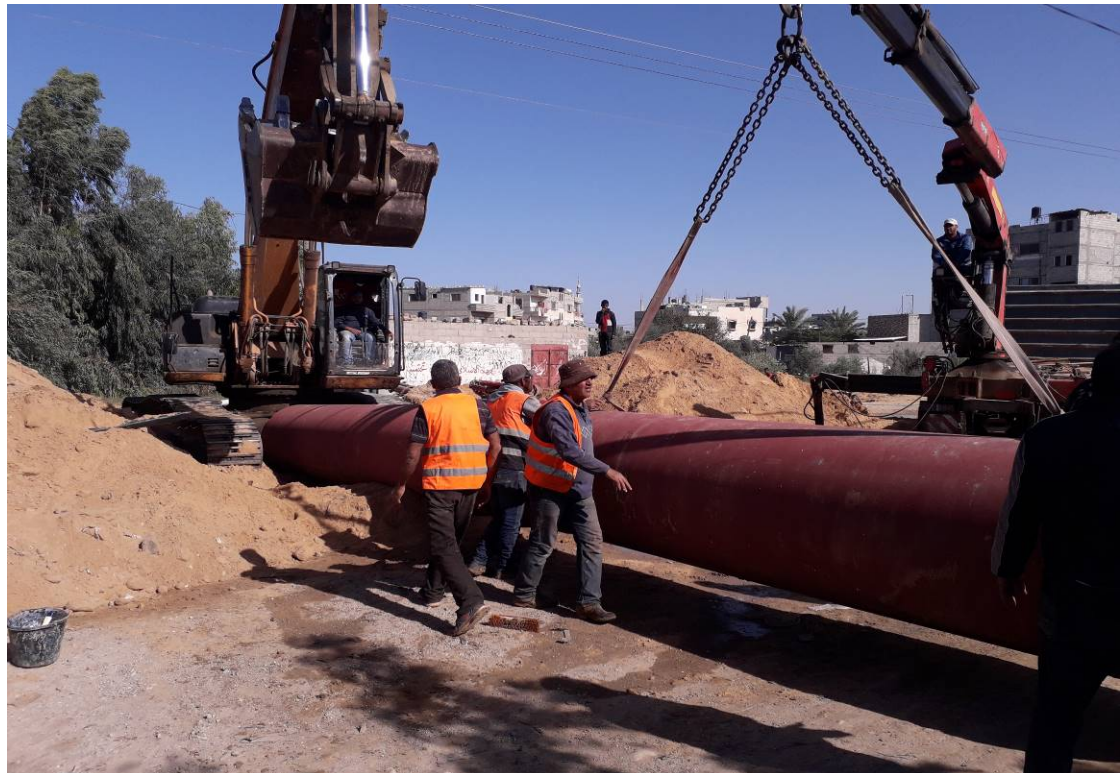
Ductile Iron Pipes Entered Gaza and Installed on Site for the Effluent Pressure Lines (CMWU Package) up to Completion in June 2020
